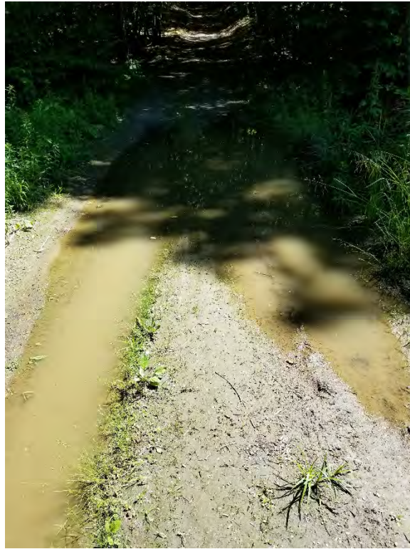
Example of drainage issues on old logging road
