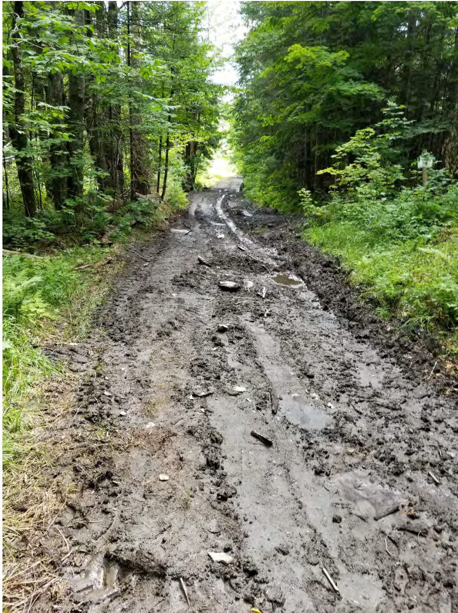
Example of drainage issues on Thompson Road
